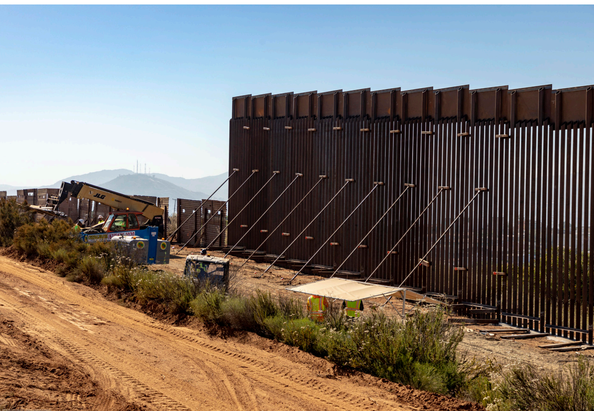
Construction crews work on the new border wall on the boundary between the United States and Mexico near the Calexico Port of Entry on June 19, 2019. Credit: Mani Albrecht for U.S. Customs and Border Protection/Flickr.
